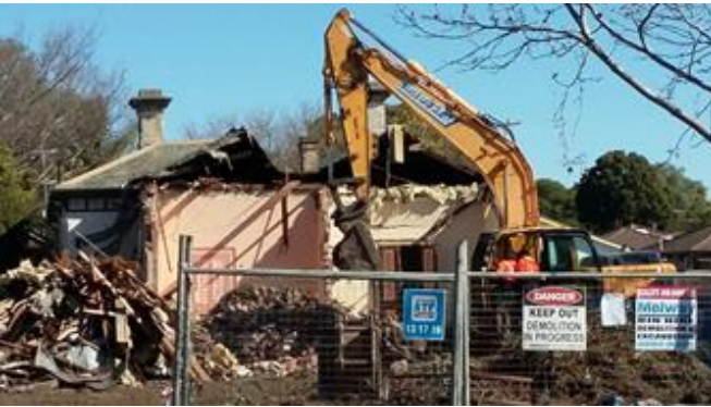
Left: Reduced to rubble: 368 Auburn Road Hawthorn (photo Liz Burton)
